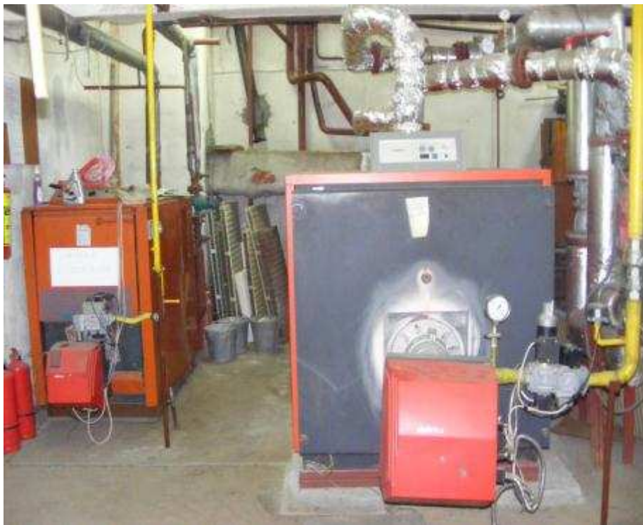
Picture 1: Boiler room
